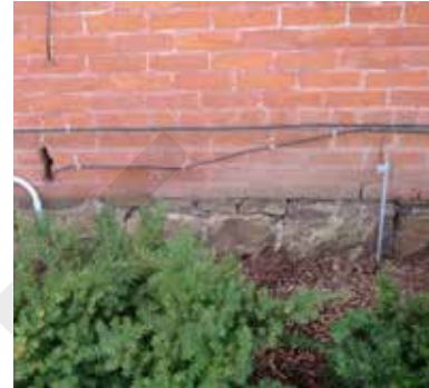
Open mortar joints in brick and stone foundation masonry (ERA, 2021).
