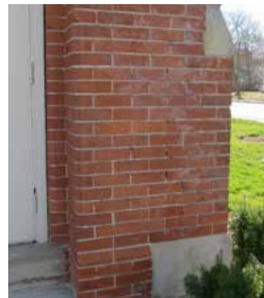
Open brick mortar joints near grade on west elevation (ERA, 2021).
