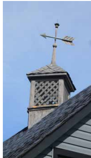
Deteriorated woodwork on roof cupola ventilation structure (ERA, 2021).
