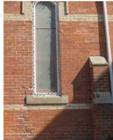
Area of deteriorated/spalled brickwork on south elevation (ERA, 2021).
