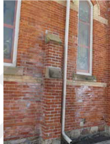
Efflorescence staining on north elevation (ERA, 2021).
