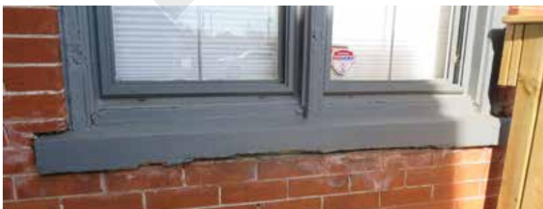
Wood rot in window lug-sill (ERA, 2021).
